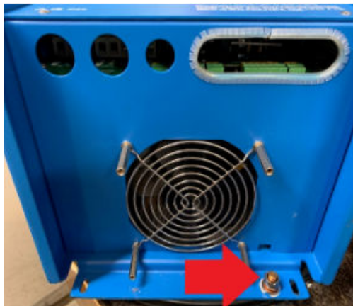
Figure 26 - 3kVA Ground Connection Point
